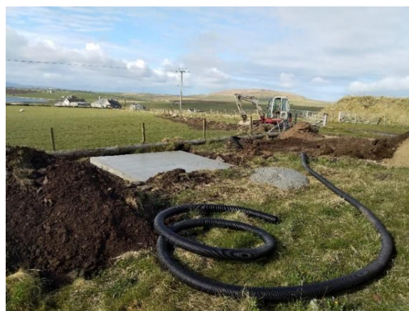
Figure 2.7: Concrete plinth for comms cabinet, with power and communications ducting laid out prior to installation.
