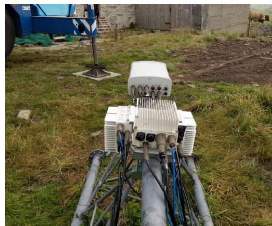
Figure 2.10: Radio equipment installed on mast.
